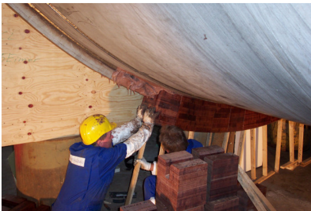
Bonding of dehonit® / Permalı fixed bearings under the world first LNG cylinder Tank
